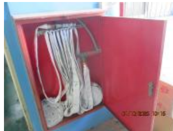
27.Outdoor fire hydrant.JPG
