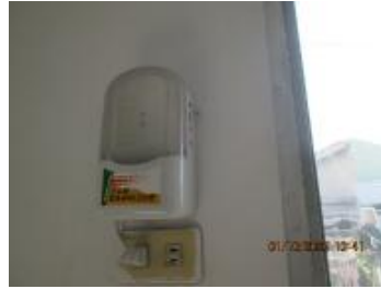
39. Foreign worker dormitory (Emergency light).JPG
