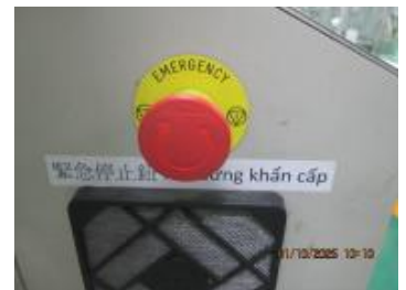
25.Emergency stop button.JPG
